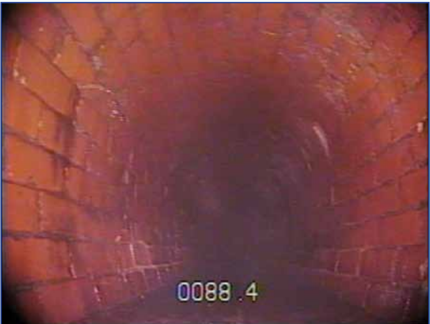
Representative image of brick storm sewer in good condition from Dedham, MA
